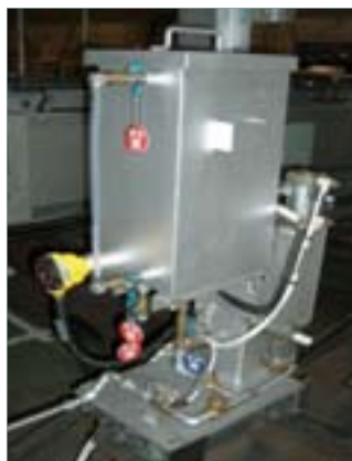
Solvent neutralizer feeder (to prevent oxidation of solvent and handle corrosion of equipment)
