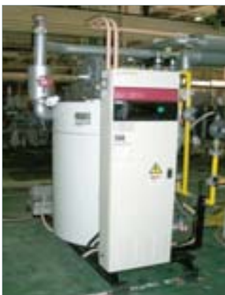
Thermal oil boiler (13 A LPG butane)
